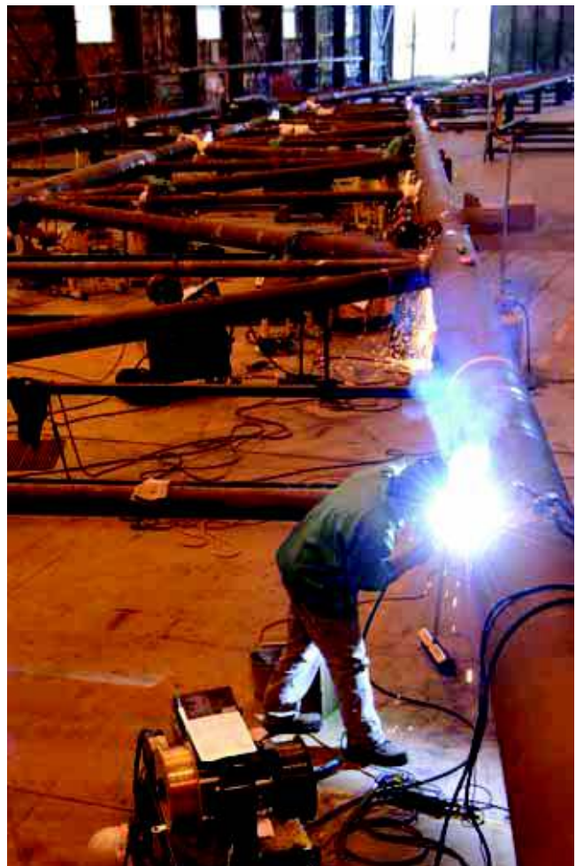
Assembly of the flare tower for the Deep Panuke production platform in Pictou, Nova Scotia
